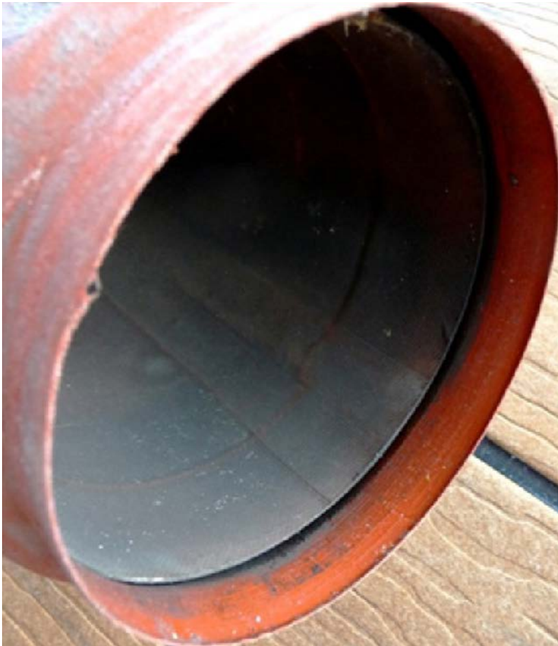
Contaminated Air Duct. Quelle: AERO
